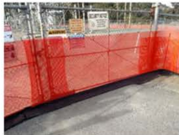
Gate Panels with Attached Ground Sweeps
