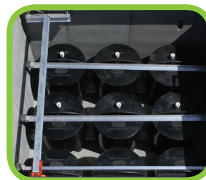
BayFilter Vault Overview
