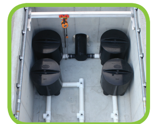
Vault Internal Assembly
