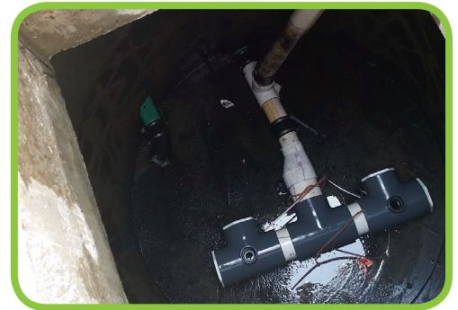
Manifold Tee View of a Cleaned System
