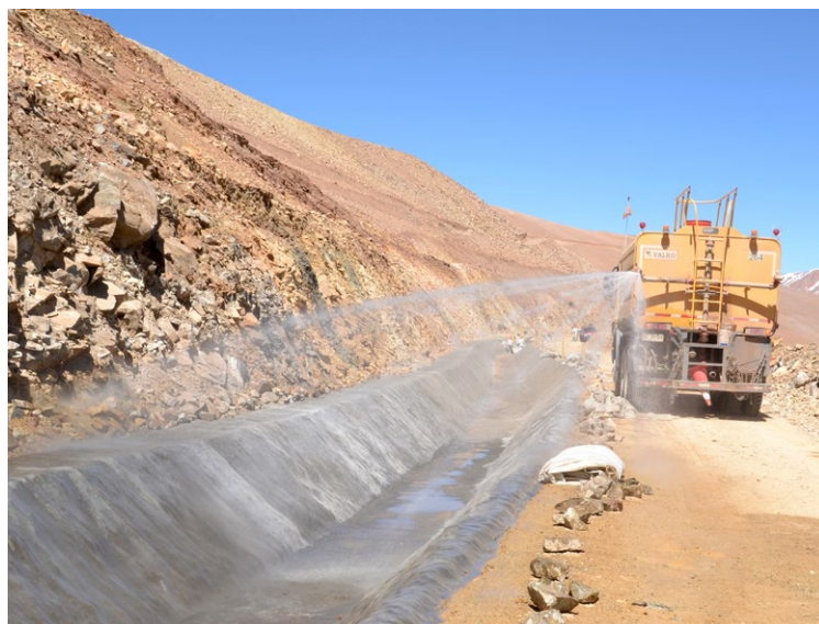
Figure 2. GCCM hydrated by spraying resulting in pooling water in the invert. These parts of the GCCM structure cure in immersed conditions.
