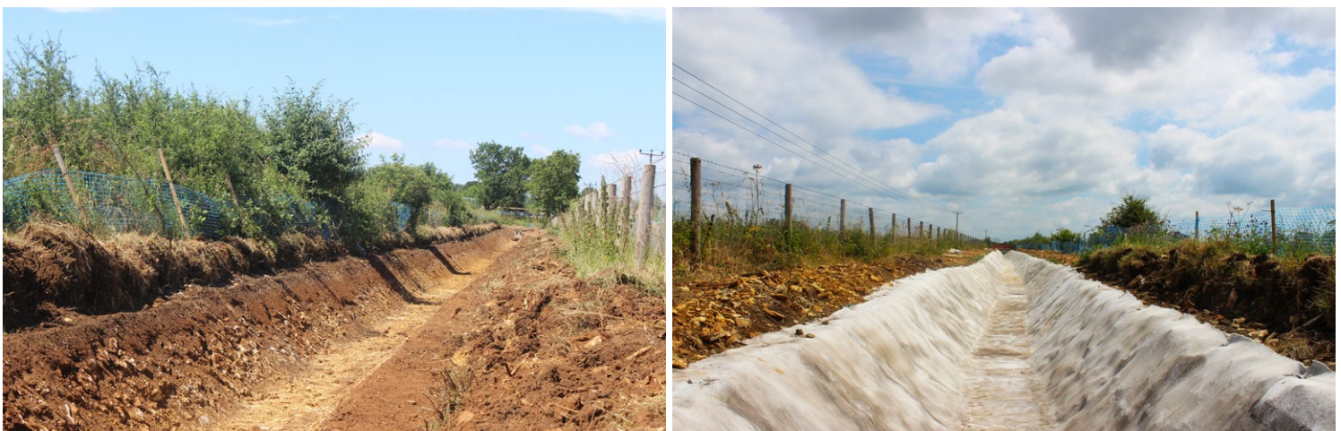
Figure 3.2 CC channel prepared with a ditching bucket (images taken before and after install)
