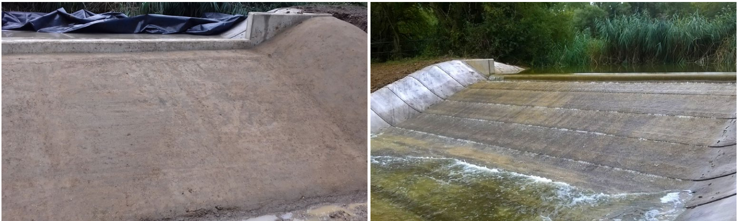
Figure 3.1 CC spillway installed on a trowelled sharp sand substrate (images taken before and after install)
