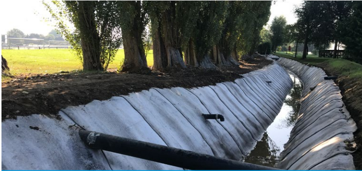
Striped appearance immediately after installation
