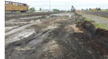
Figure 1. View of the site showing poor ground conditions
