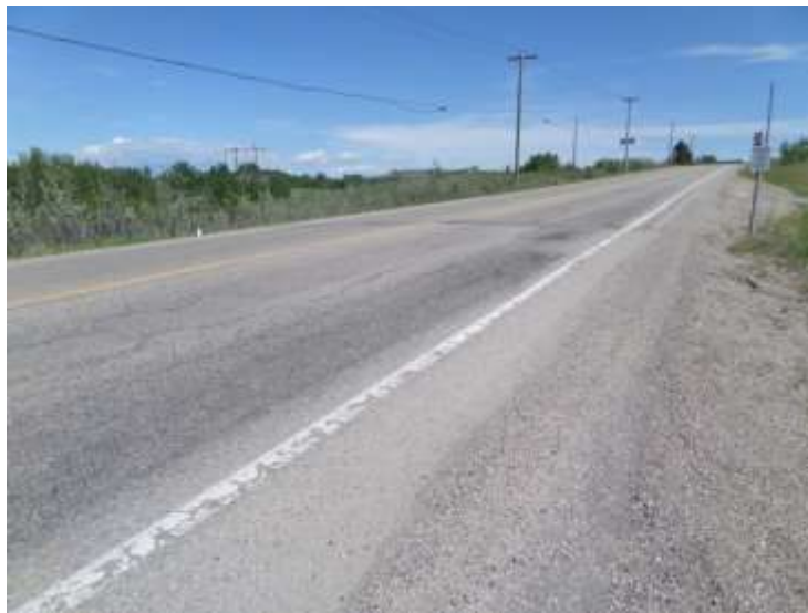
Figure 2 - General pavement condition on 101 Street
