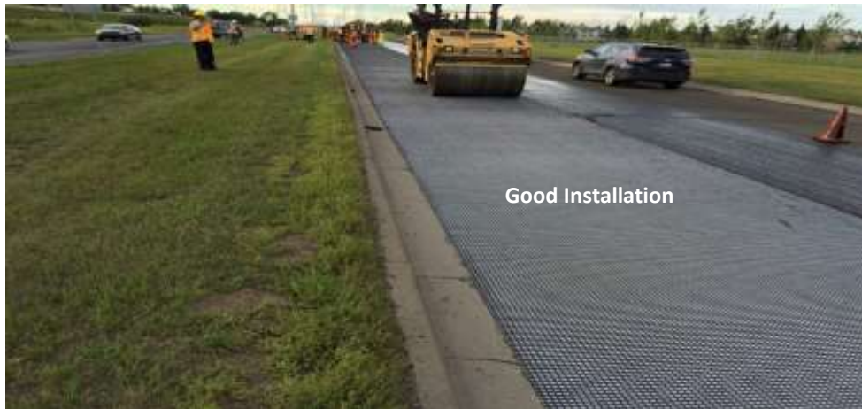
Figure 4 - Sarcee Trail Grid Installation – well placed and bonded
