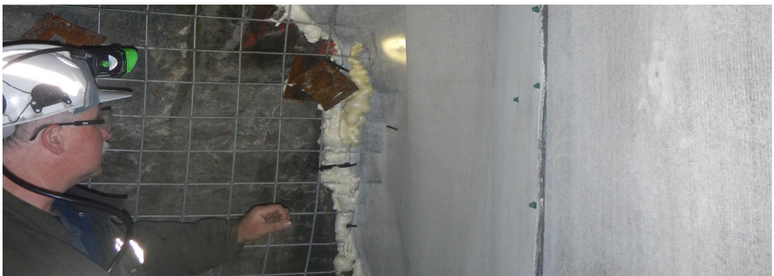
Spray foam used to fill any voids between vent wall and surrounding rock
