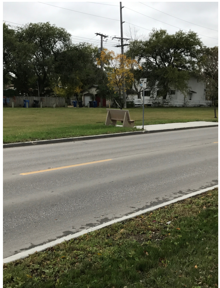
Completed construction with Spartan Road Grid™ 10C showing no trans cracks after 2 years.
