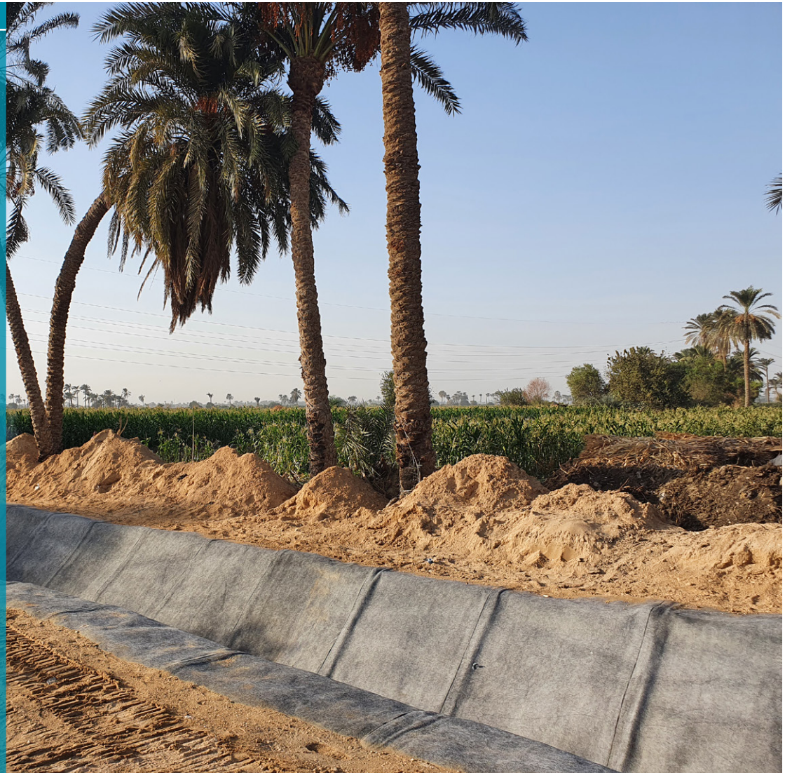
Completed CCX-B TM trial installation in Egypt
