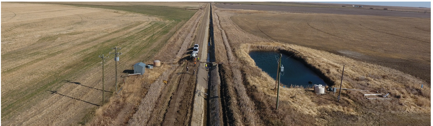
Bird's eye view of the CC installation process otop of the existing damaged concrete channel
